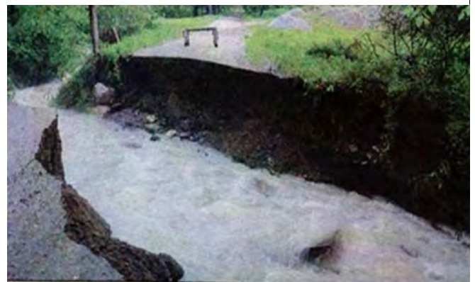
Fig. 3.2.5. Treadwell Hollow Road crossing (upper photo); streambank and infrastructure damage Hemlock Brook
