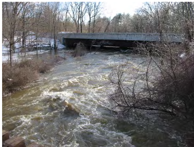
Fig. 3.2.8. Route 7A bridge floods 3/08/2011
