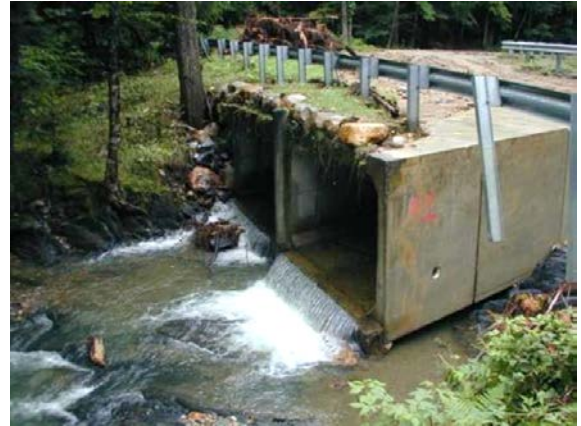
Bridge in Worthington had history of failing. In 2003 road washed out and was closed to all traffic.
