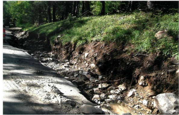
Fig. 3.9. T.S. Irene flooding along Middlefield Road caused severe erosion of soils, washouts of partially laid drainage ditches and undermined and broke up the edges of newly laid blacktop
