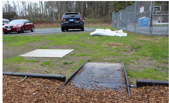
The town installed a transition to provide ADA access to the newly constructed playground.
