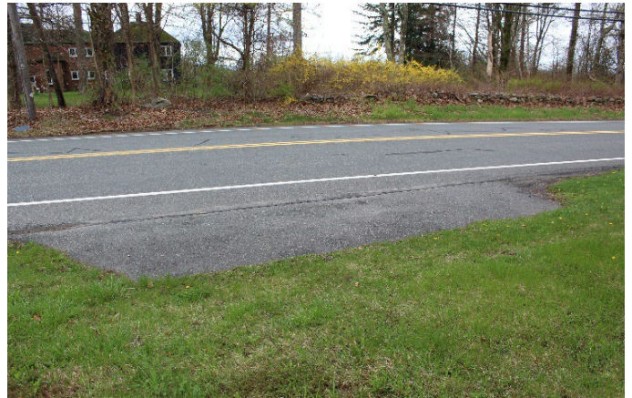
There is a small area to park but it is not lined and there is no signage to provide accessible parking.
