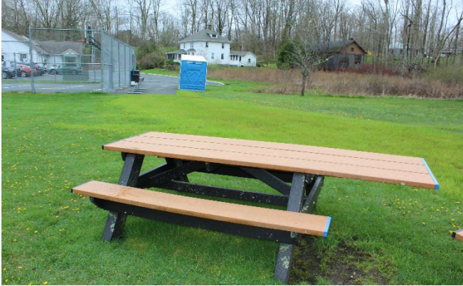
The park had ADA picnic tables and accessible restroom but there is no pathway connecting the two elements.
