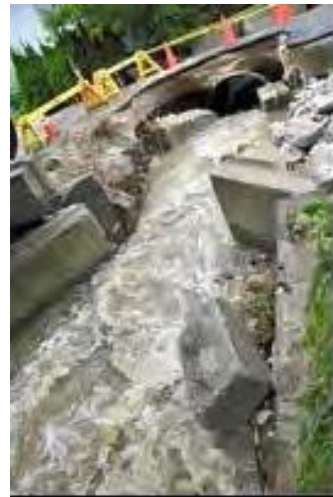
Damage to Davis St. Bridge 9/11/2018 (photo courtesy of the Berkshire Eagle)
