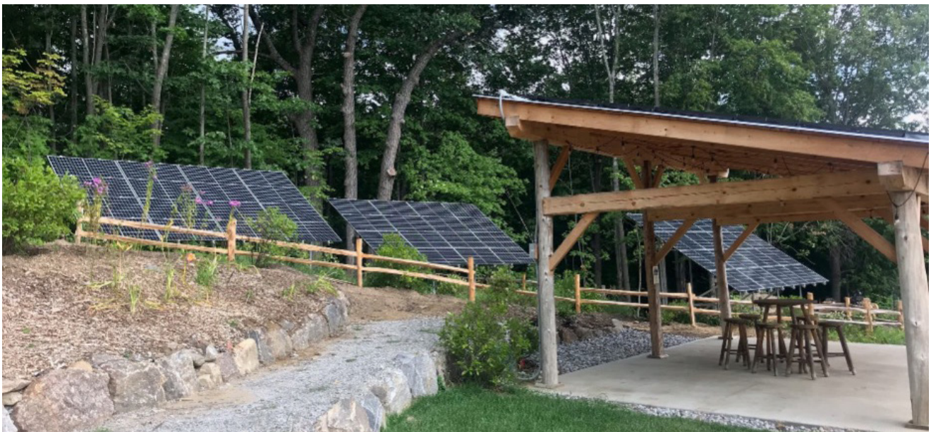
Above: The NH Solar Shares site in Plymouth NH doubles as a public park.
