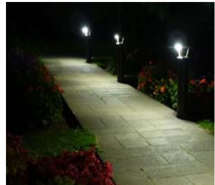
Figure 5.9 Solar Powered Bollard Lights
