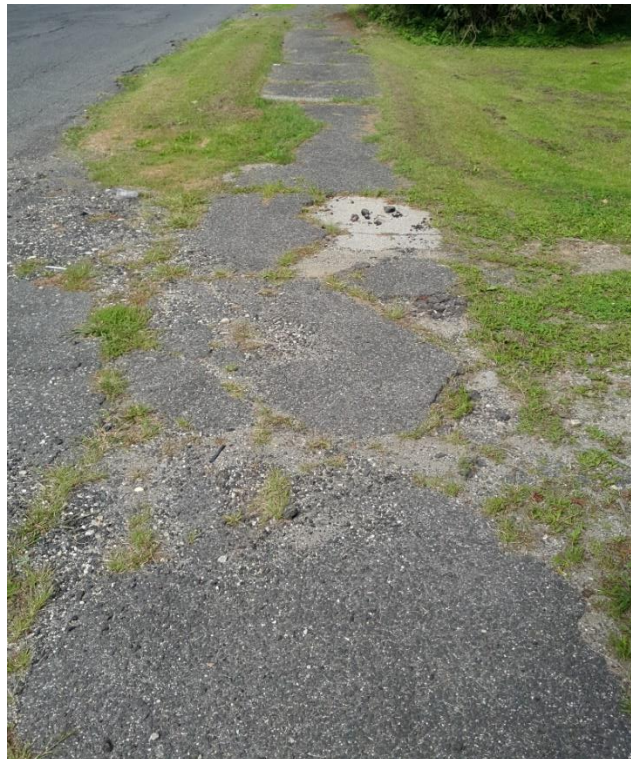
Figure 13. Sidewalk on Church Street in Poor Condition
